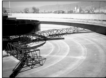
Figure 2 Picture of the (empty) Central Davies clarifier
