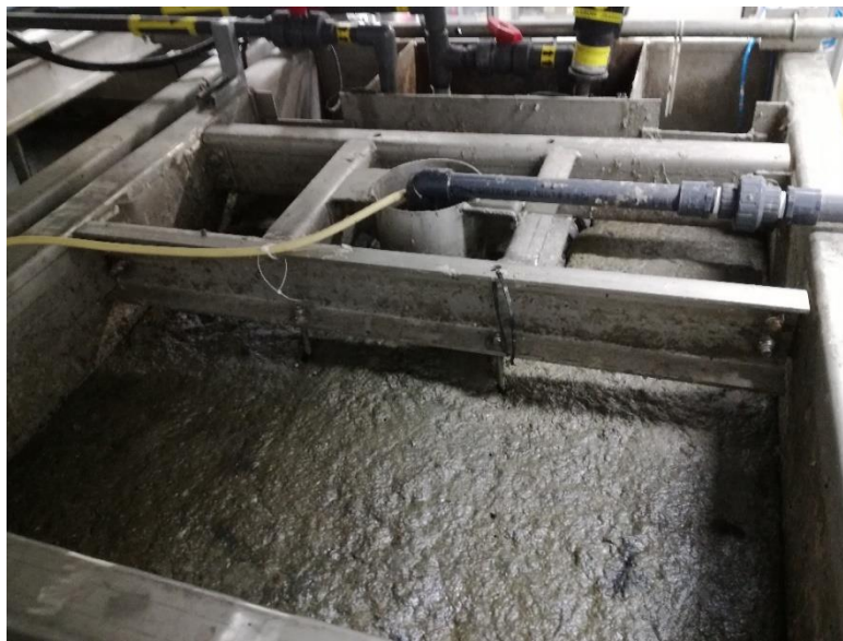
Figure 29: Rising sludge on the primary clarifier on Day 4 (Stage #6).
