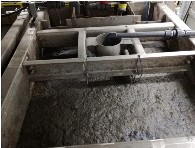
Figure 21: Rising sludge on the primary clarifier on June 11 (Stage #4).
