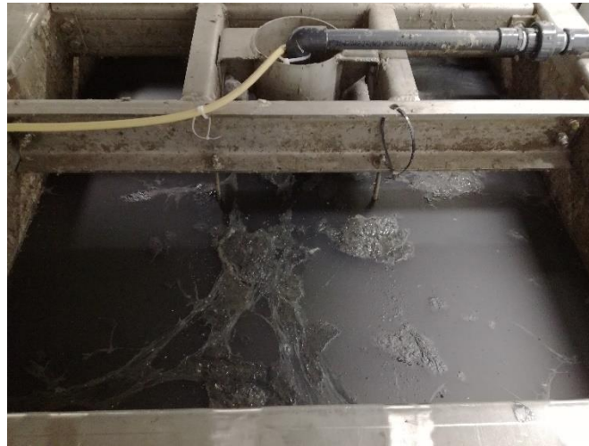
Figure 74: Film on the clarifier's surface after \text{NaHCO}_3 dosage.
