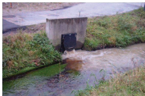
In many cases, implementing control can reduce the numbers of combined sewer overflows.
