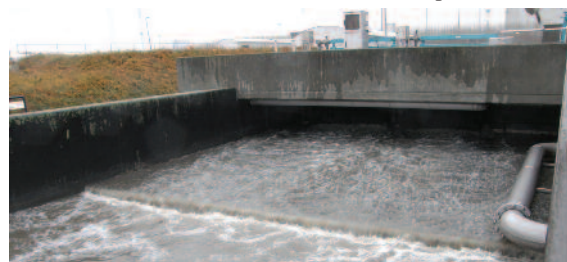
Lynetten wastewater treatment plant in Copenhagen, Denmark. When the hydraulic capacity of a WWTP is exceeded, bypass gates are opened. Integrated control minimizes the need for bypass.
