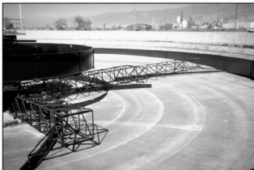
Figure 3 Empty settler with baffled centre well
